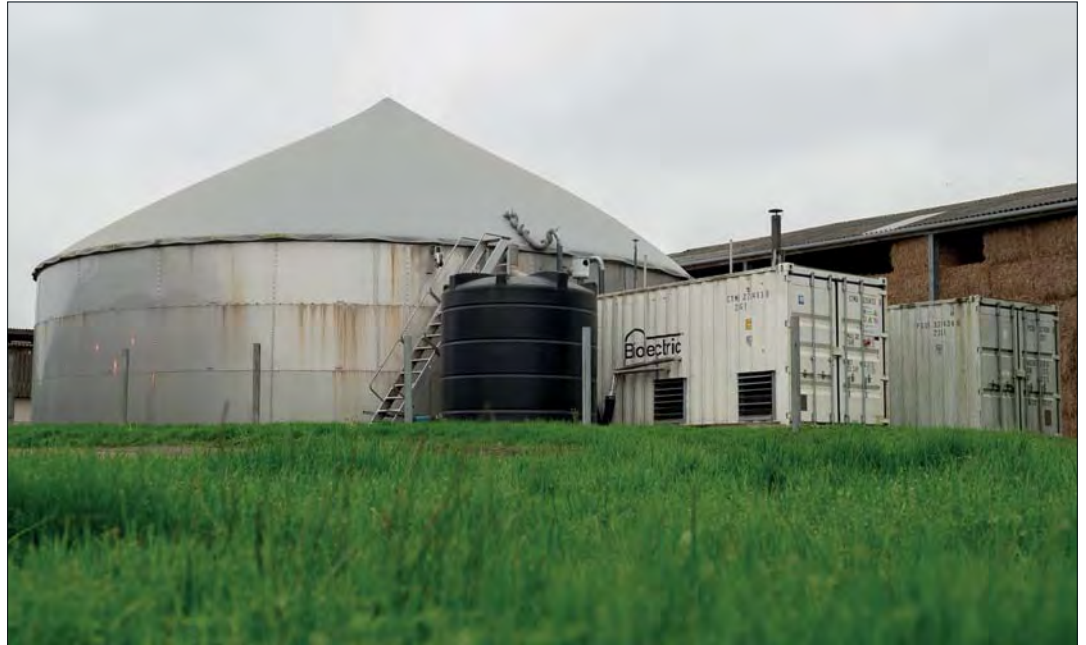
Slurry from the dairy cows is used to power a micro anaerobic digester, which produces electricity and digestate
